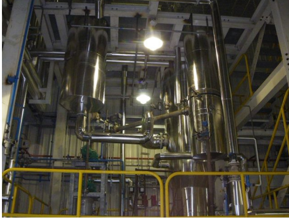
Oil Recovery Plant
