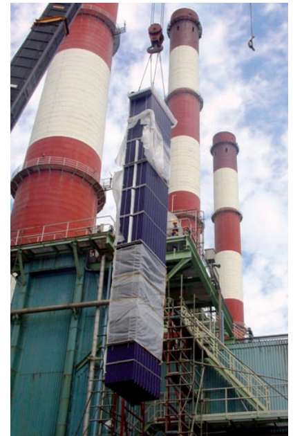
Power plant, 3 blocks with a capacity of 500 MW each
