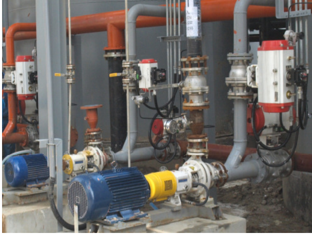
Pumping Station for Chemical Additives
