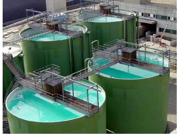
Brine Purification Plant
